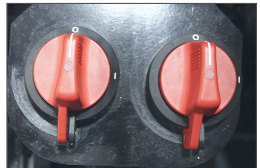
Figure 10. Switches in off position
