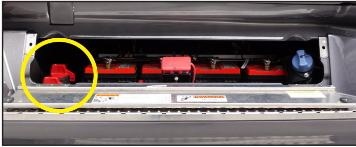
Driver step hatch with battery bank and disconnects
