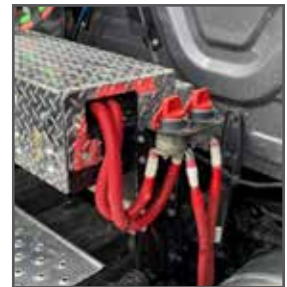
Figure 12. Passenger-side battery disconnects
