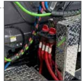
Figure 13. Driver-side battery disconnects
