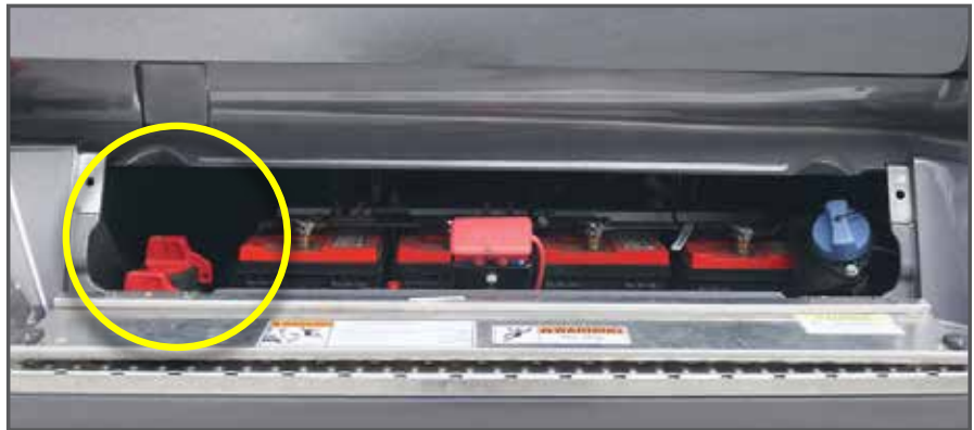
Figure 8. Driver step hatch with battery bank and disconnects
