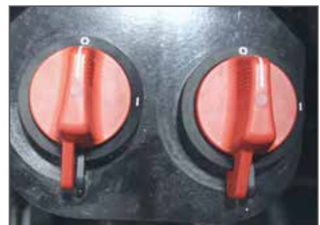
Figure 10. Switches in off position
